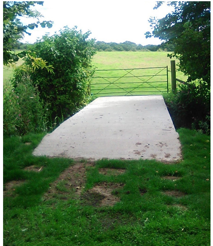
One work party from Mountjoy rebuilt our bridge into the main sheep field, despite inclement weather (rain) we managed and the bridge is here.
